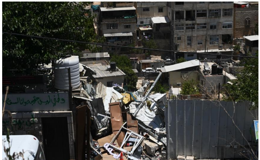
Shop demolished by Israeli authorities, Silwan, East Jerusalem. 29 June 2021. ©OCHA
