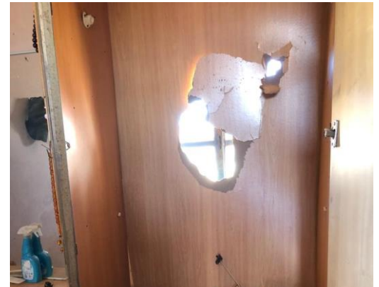
Damaged door from Umm Fagarah settler attack. ©Photo by OCHA
