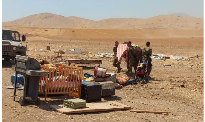
Demolition in Humsa Al Bqai'a, 7 July, photos by the community for OCHA
