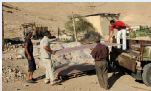
Save the Children UK and its local partner renovated houses for 30 families in the Jordan Valley as a means to prevent forced displacement. PHOTO/Hiba Qaraman
