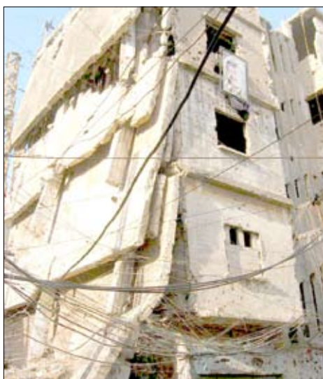
A destroyed building in Burj el Barajneh camp, Lebanon. (© Courtesy of al Najda Association)
