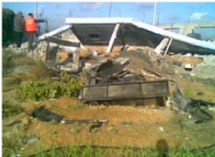
Damages to Gaza Waste Water Treatment Plant, picture provided by CMWU
