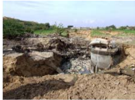
Damages to Khadiga Well , picture provided by CMWU
