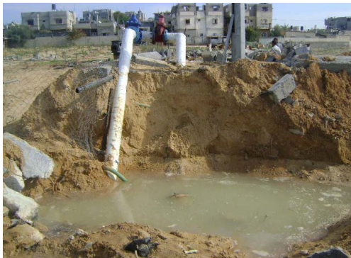
Khadeeja well before repairs, picture provided by CMWU
