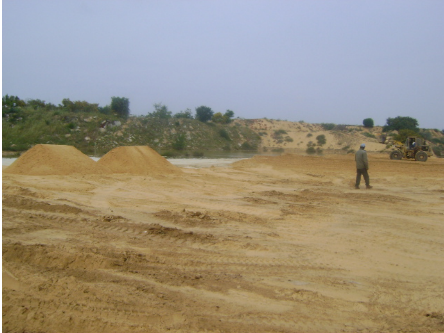
Figure 8 Sand being positioned by the CMWU contractor at the stationery leading edge of the escaped wastewater (Photograph by CMWU, received by WASH Cluster Team on 6 th April 2009)
