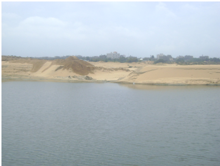
Figure 10 Existing pond and the opening at the embankment; CMWU contractor completing repairs to the temporary disposal ponds (Photograph by the CMWU on 2 nd April 2009)
