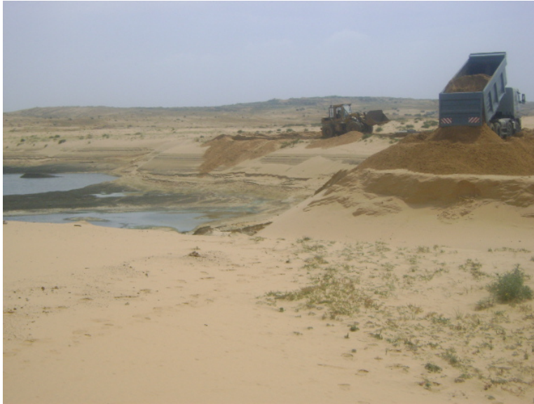
Figure 11 CMWU contractor completing repairs to the temporary disposal ponds (Photograph by the CMWU on 2 nd April 2009)
