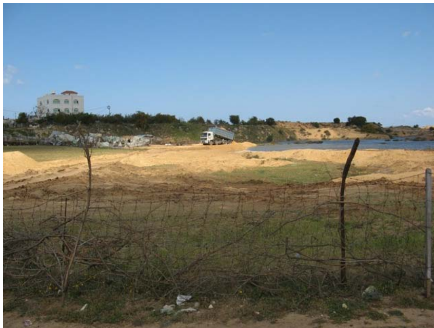
Figure 5 Sand being dropped by the CMWU contractor at the stationery leading edge of the escaped wastewater (Photograph by the WASH Cluster Team on 29 th March 2009)
