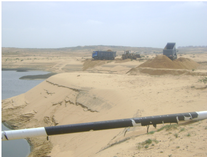
Figure 12 CMWU contractor completing repairs to the temporary disposal ponds (Photograph by the CMWU on 2 nd April 2009)
