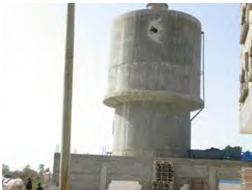
Damages in water tank
