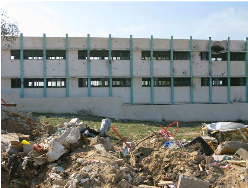
Damages to the only school in Wadi Gaza
