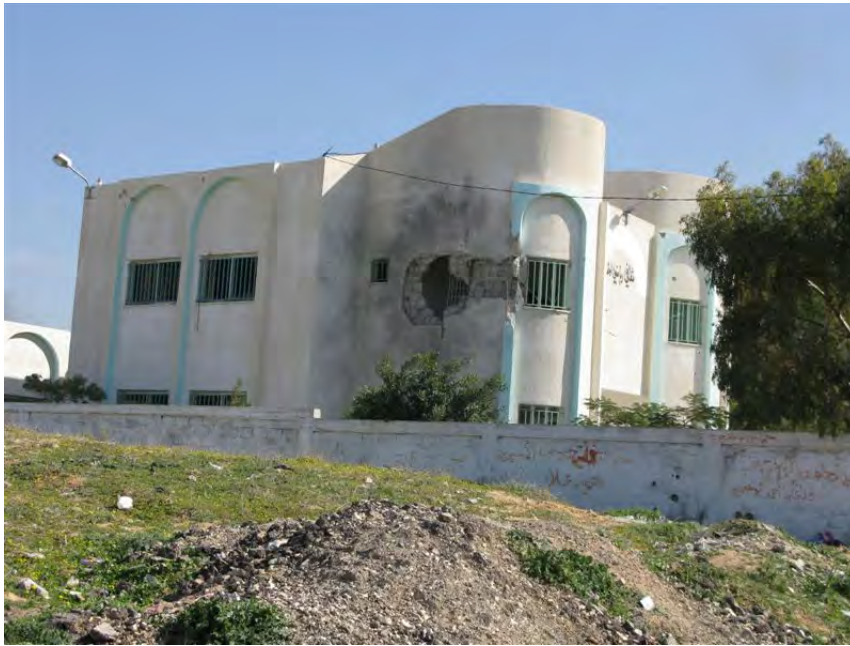
Damages to the Cultural Center
