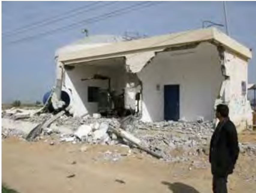
Damages to the generator and storage rooms
