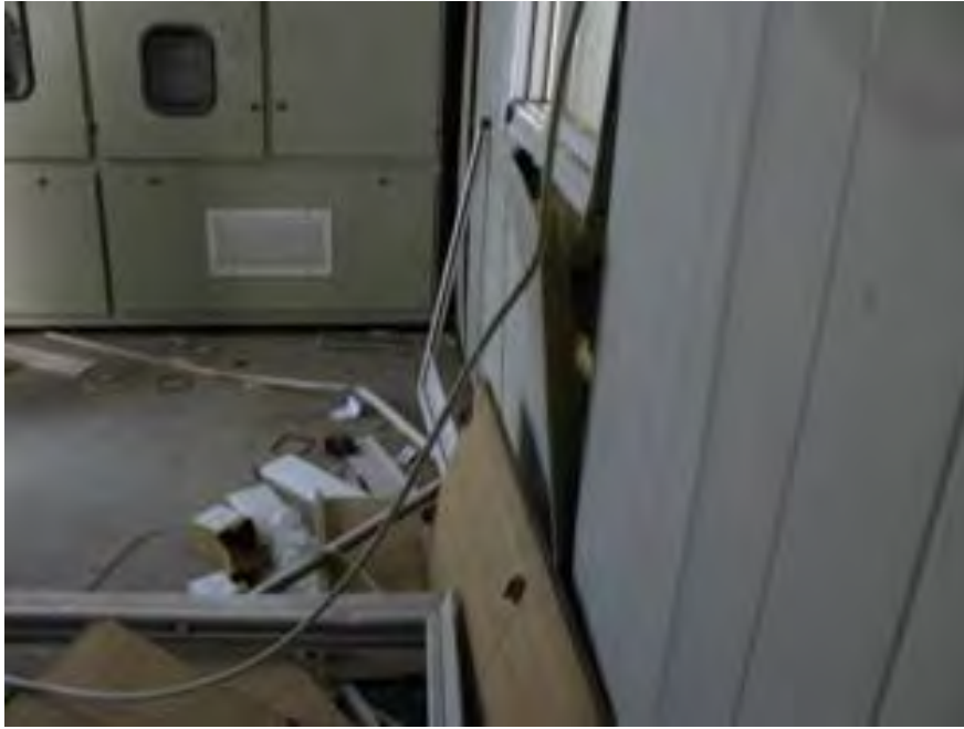
Damages in water well control room
