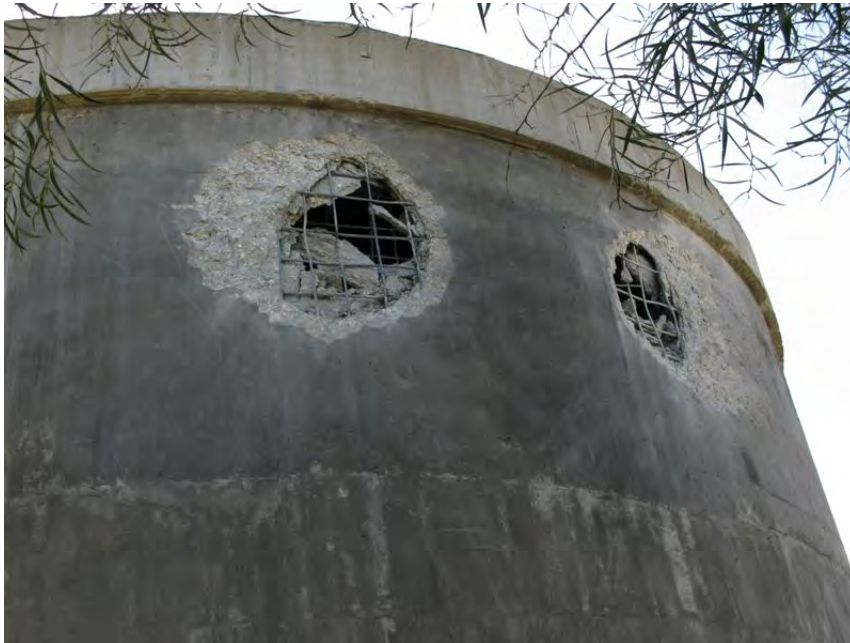
Damage to the Water Tank
