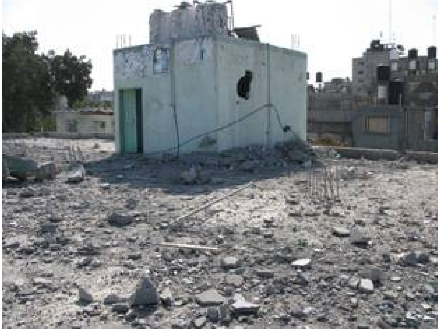
Debris from the nearby mosque on the clinic's roof, the damaged staircase and water tanks
