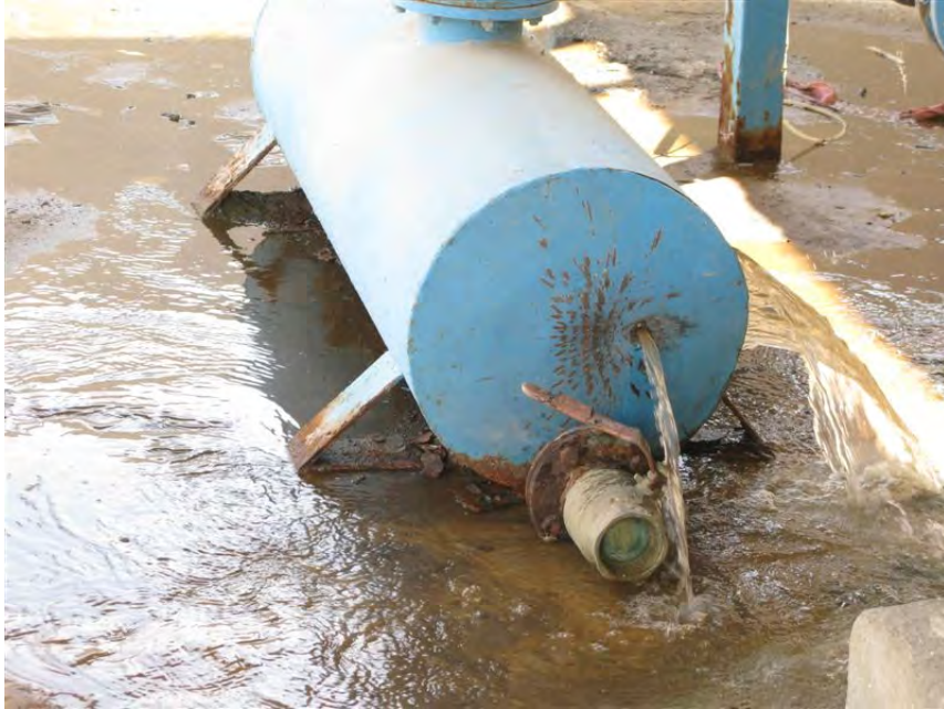
Damage to the water cyclone at the water well
