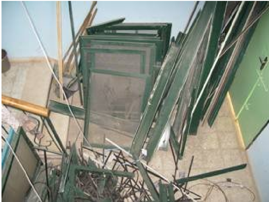
Damages to the clinic's aluminum windows
