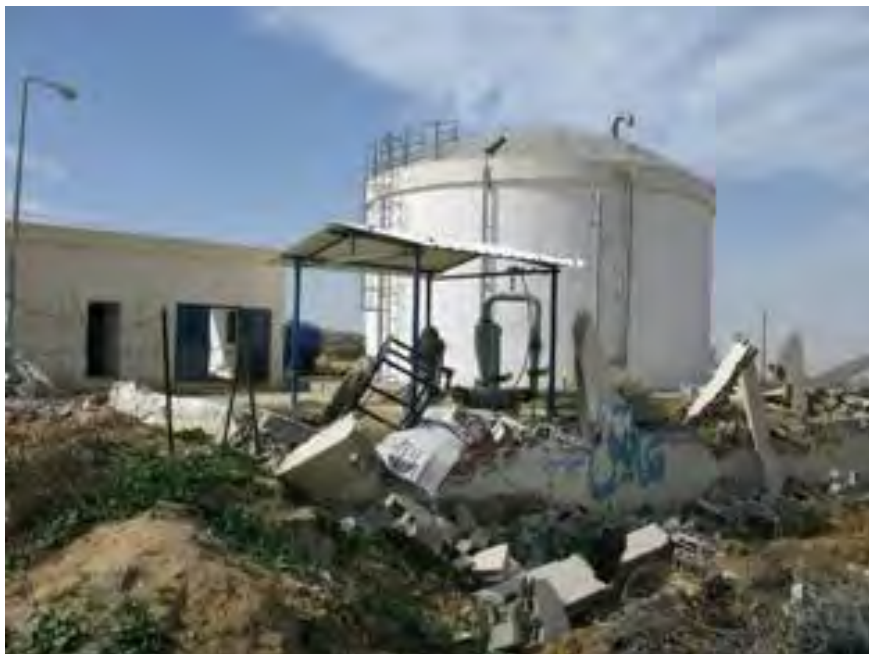
Damages to water tank & well
