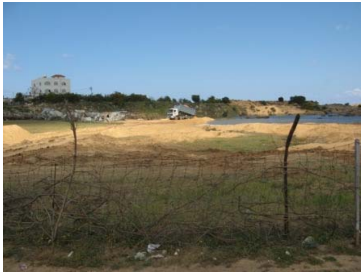
Figure 5 Sand being dropped by the CMWU contractor at the stationery leading edge of the escaped wastewater (Photograph by the WASH Cluster Team, Sunday 29 th March)
