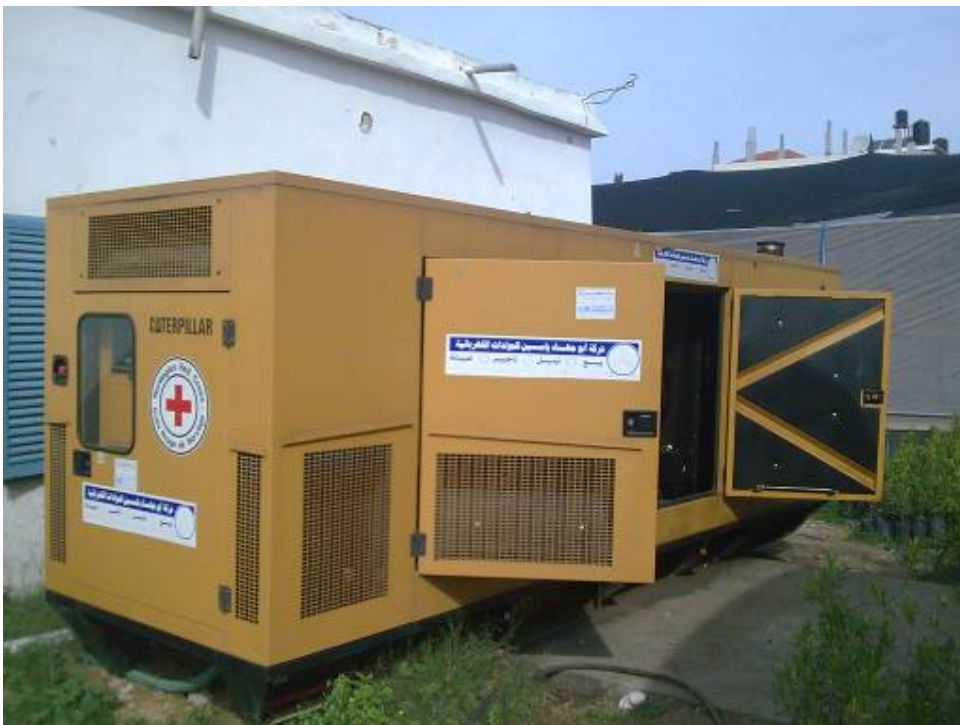
Generator supplied with diesel fuel for a well in Al Sheikh Redwan – Gaza city (19/01/09)
