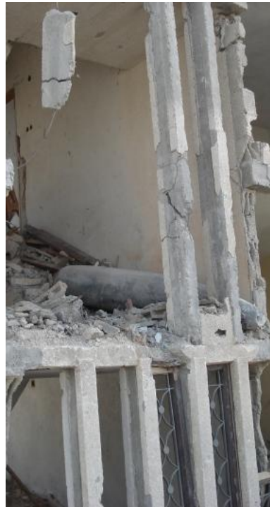
An unexploded 2000lb bomb on the second storey of a damaged building in Rafah, Gaza Strip
