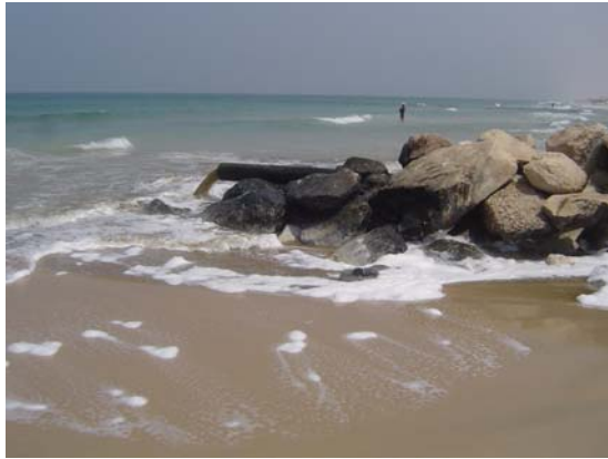
Partially treated sewerage discharging into the sea, Swedish Village, Rafah (credit: Tim Forster)
