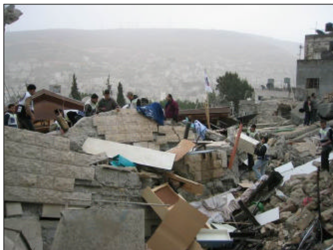
Demolished building in south west Nablus – OCHA Jan 2004
